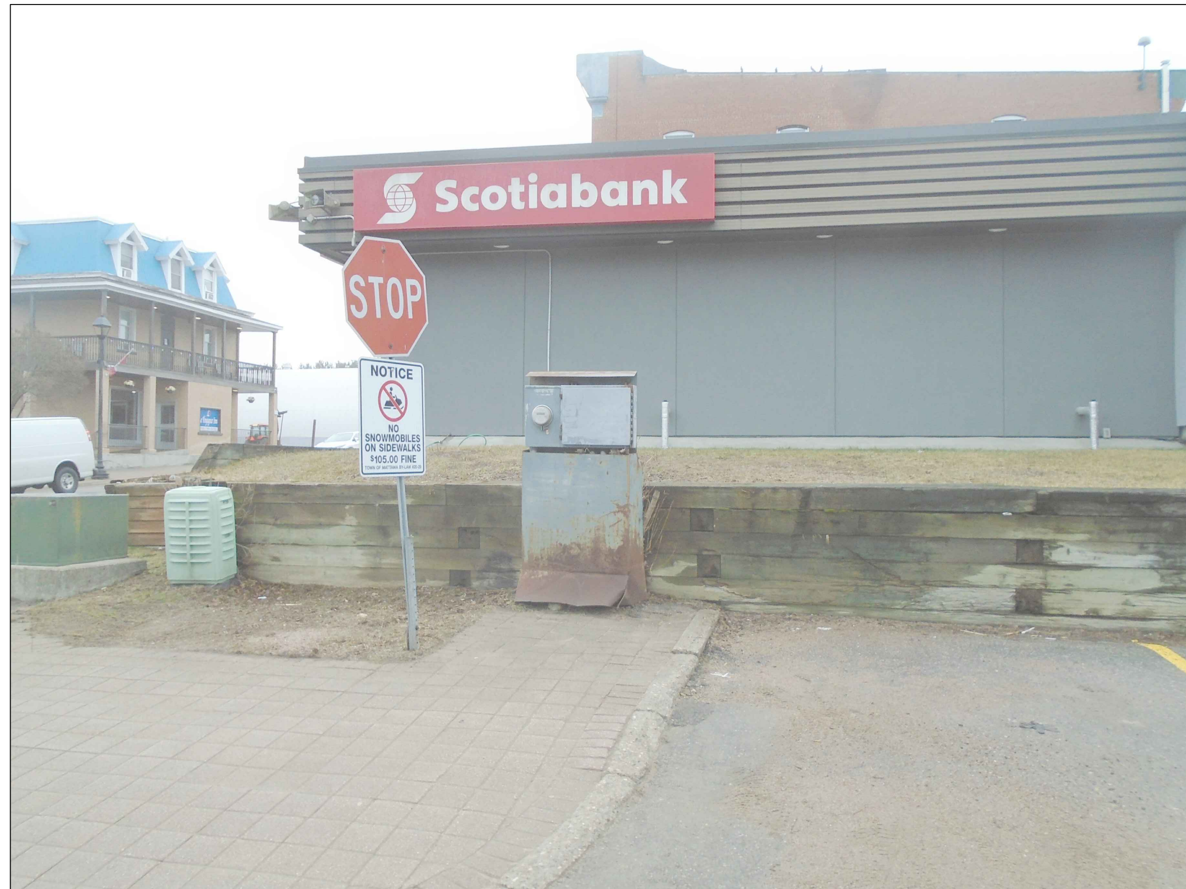
EXTERIOR BREAKER PANEL
