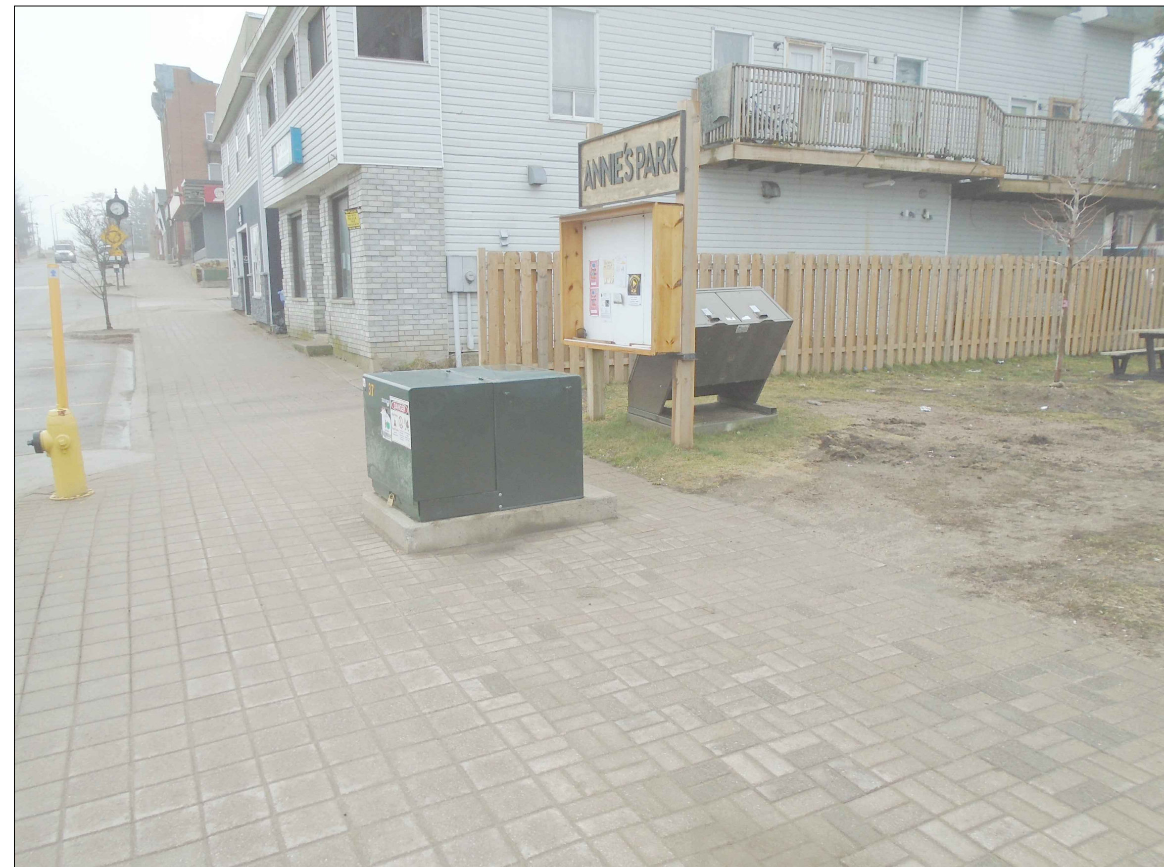
HYDRO ONE TRANSFORMER
